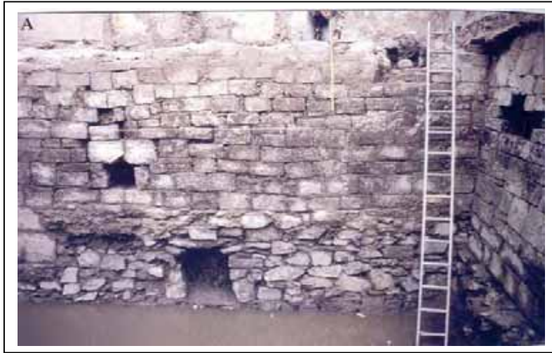
The city wall at 81-83 Grand Parade/St. Augustine Street. This length of wall was rebuilt in the eighteenth century as a quay wall.
